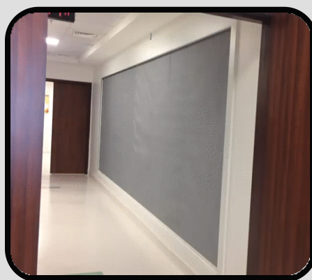
Kent Fire Curtains Jeddah Hospital
